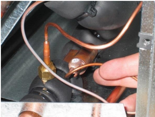
Figure 28. Thermal Measuring Bulb Placed on Copper Tube.
